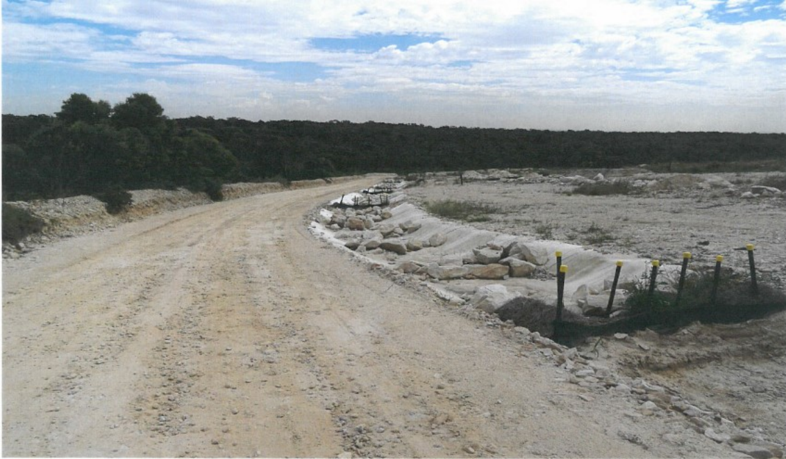
Figure 1 Lined drain along western perimeter haul road with siltation traps
